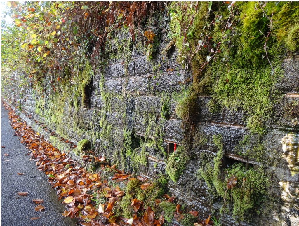
Plate 2: Close up of wall shown in Plate 1, note bricks being eroded by water and moss
